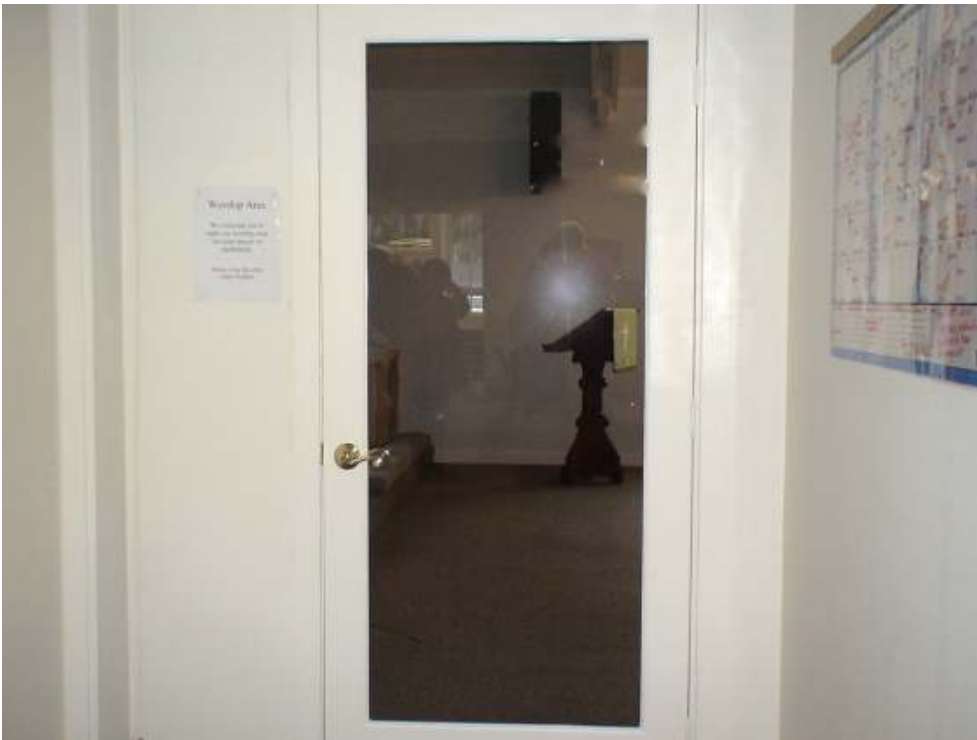
New glass door to worship space from the meeting hall installed; replaces old worn solid wood door.
